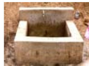
Faucet where water flows by gravity from the spring-capture box.
